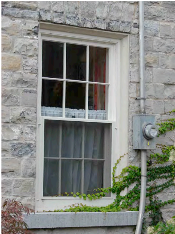
Six over Six Paned Heritage Window on Earl Street Façade/ Paul Christianson 2010
